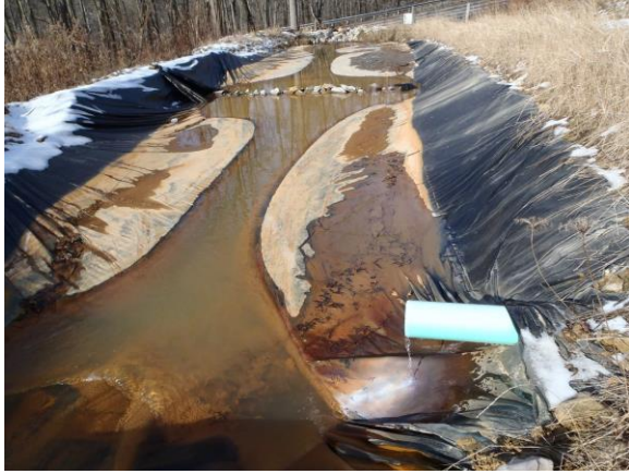
Figure 4: The liner in lined ponds may be pushed away from the soil by ground water underneath the liner, decreasing the volume and retention time in the pond.
