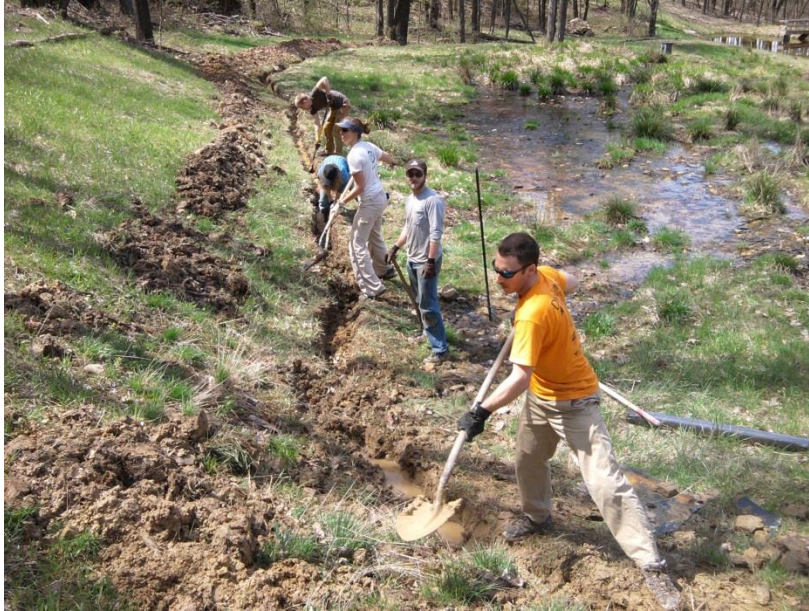
Picture 4: Friends of Deckers Creek Shovel Corps installs a French drain to prevent ponding on top of a sulfate reducing bioreactor.
