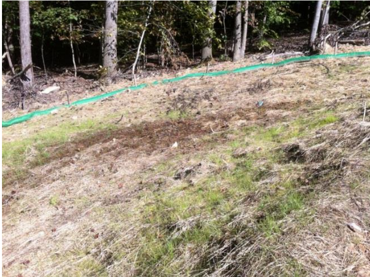
Figure 6: A spring forming during construction on a smoothed and re-vegetated slope.
