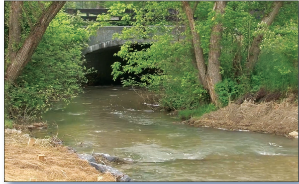
Figure 3. The stream channel was configured to allow water to flow more directly into the culvert.
