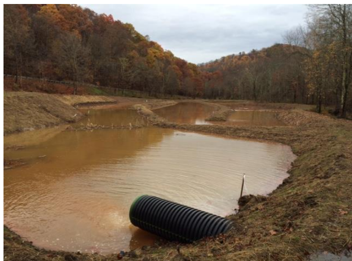
Figure 17. View of the wetland treatment cells taken during the 2015 EPA tour
