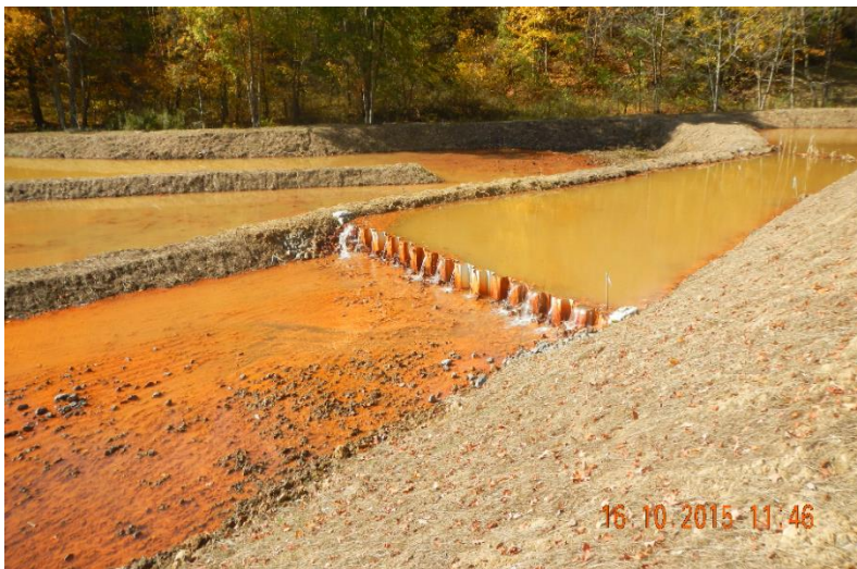
Figure 16. Aeration weir at Site 7 in wetland cell #1
