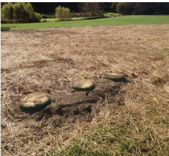
Figure 13. Shown here are the risers of the Denitrifying system installed at Poor House Farms. Tuscarora Creek can be seen in the background.
