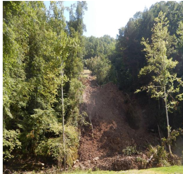
Picture 8 Oil and gas Pipeline Slip
