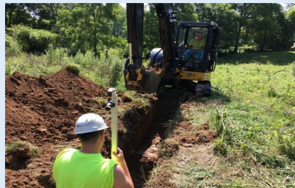
Pipeline being installed on grade along Milligan Creek in the Bungers Mill area.
