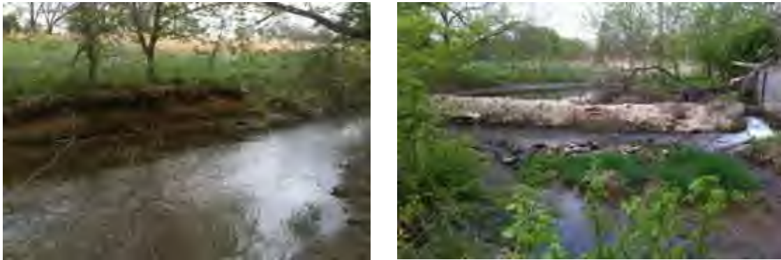
Eroding banks and dam at the stream restoration project site pre-construction.
