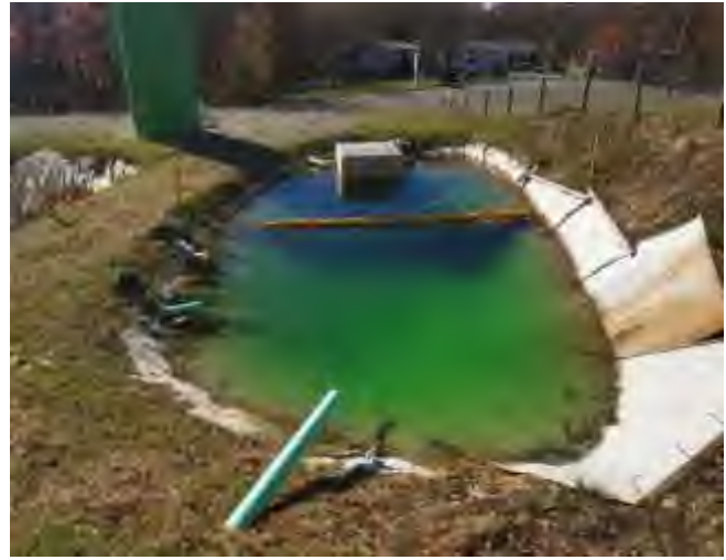
VH3 settling pond #1 and mixer
