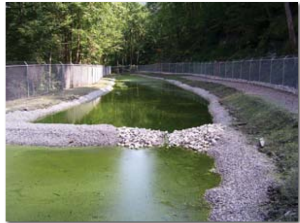
Figure 2. The Upper Mainstem Morris Creek treatment system includes a drainage channel lined with limestone.
