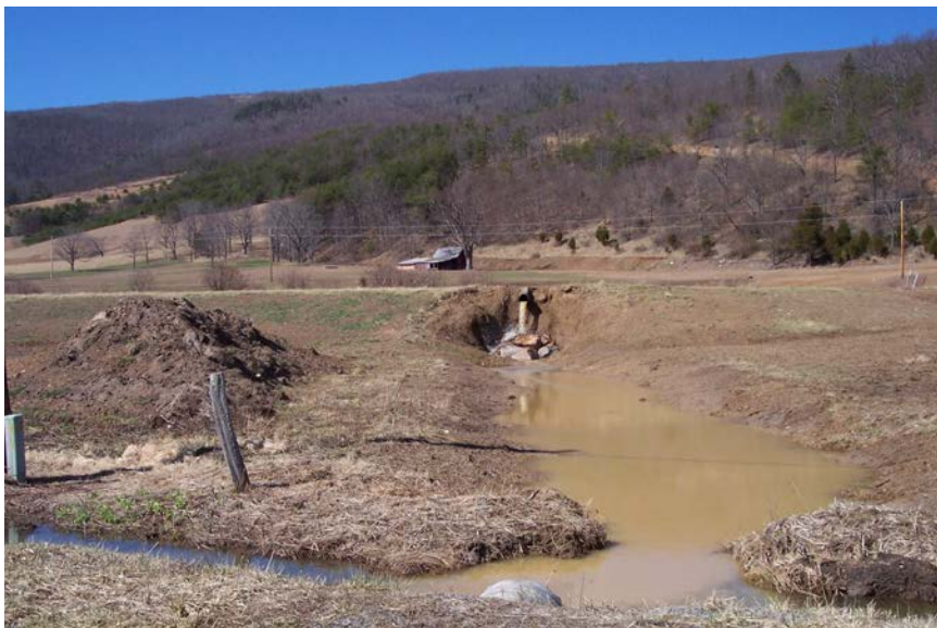
A newly constructed pond in Potts Creek discharging mud. (March 2011)
