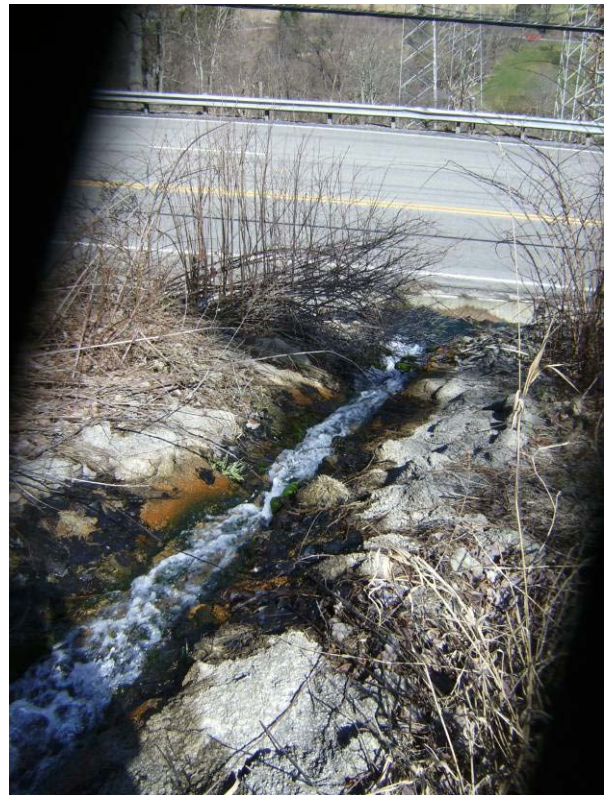
Figure 20: This photograph shows the Easton Right Portal discharge.
