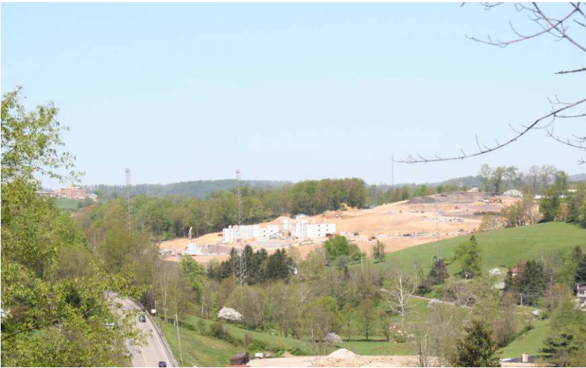
Figure 26: Development above the poorly constructed retaining wall.
