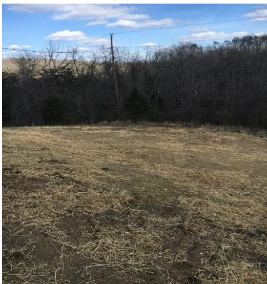
NPS 1583 post-construction. A full septic replacement has taken place. All operations of the project were coordinated by the Project Manager
