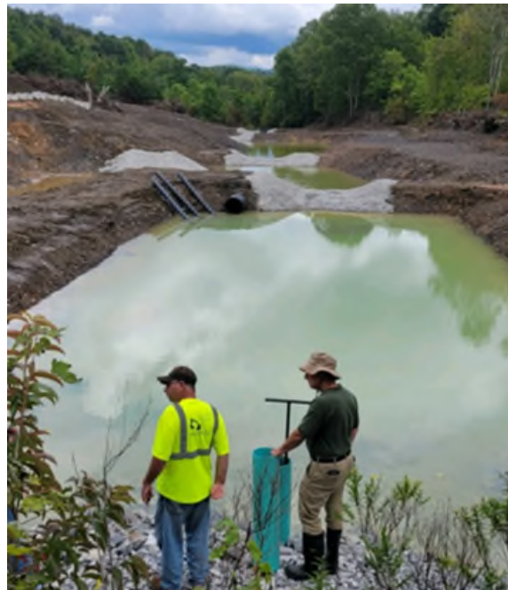
AL CON construction manager and Martin evaluate the treatment systems constructed at the Roaring Creek project.
