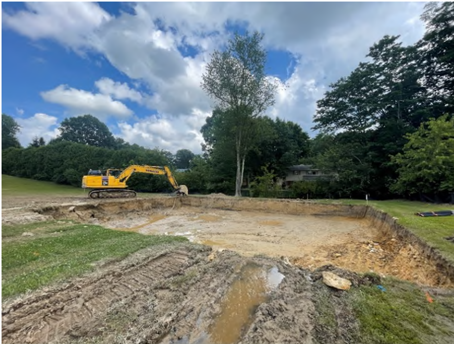
The construction site at Crescent Elementary, where the stormwater detention system will be located.
