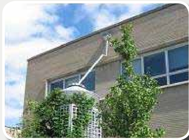
Disconnection to Rainwater Harvesting Apparatus Cistern (Source: U.S. EPA)
