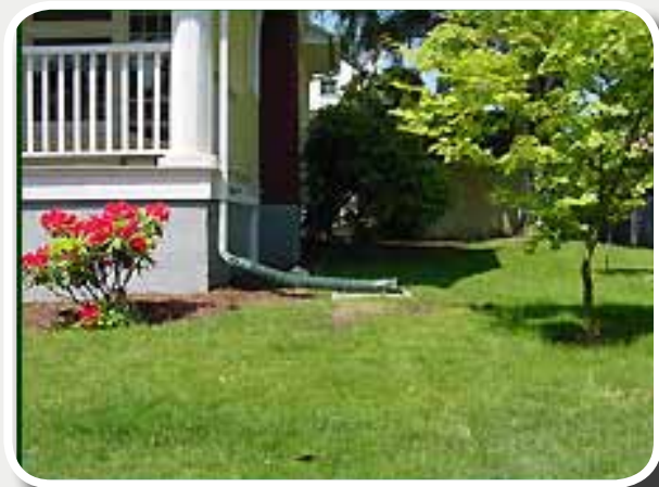
Simple Rooftop Disconnection
