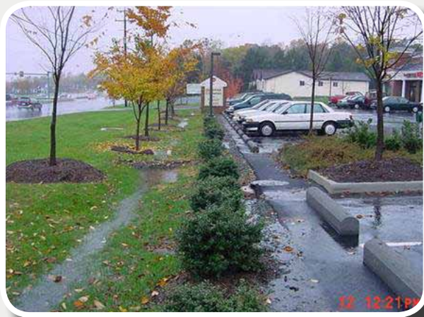
Water Quality Swale at edge of parking lot
