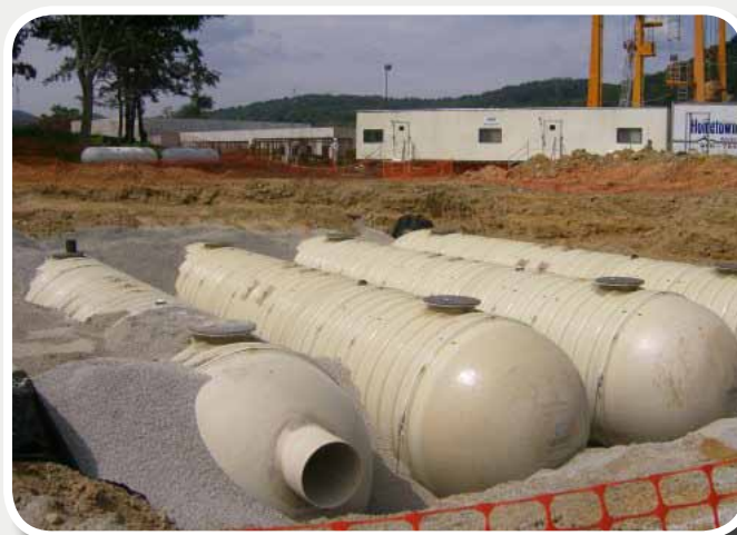
Figure RH-15. Example of Multiple Fiberglass Cisterns in Series (Source: Rainwater Management Solutions)
