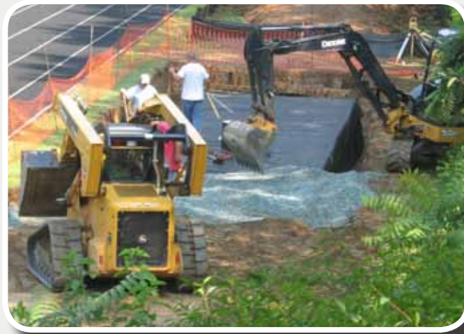
Underground Tank to Irrigate Turf Fields Source: City of Charlottesville, VA
