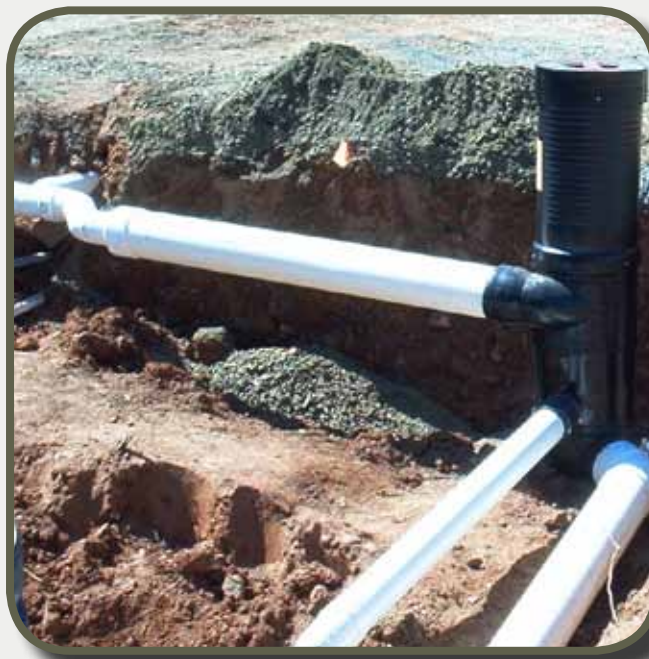
Figure RH-14. Installation of Vortex Filter prior to backfill. (Source: Rainwater Management Solutions)
