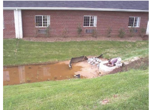
Bioretention area does not drain because of improper soil media, soils compacted during installation, and/or filter fabric under media.
