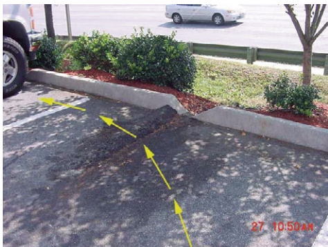
Site runoff by-passes bioretention swale because of small elevation changes during construction.
