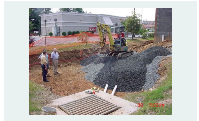
Figure 8.5. Co-inspections by construction inspectors and plan reviewers can help resolve BMP installation issues
