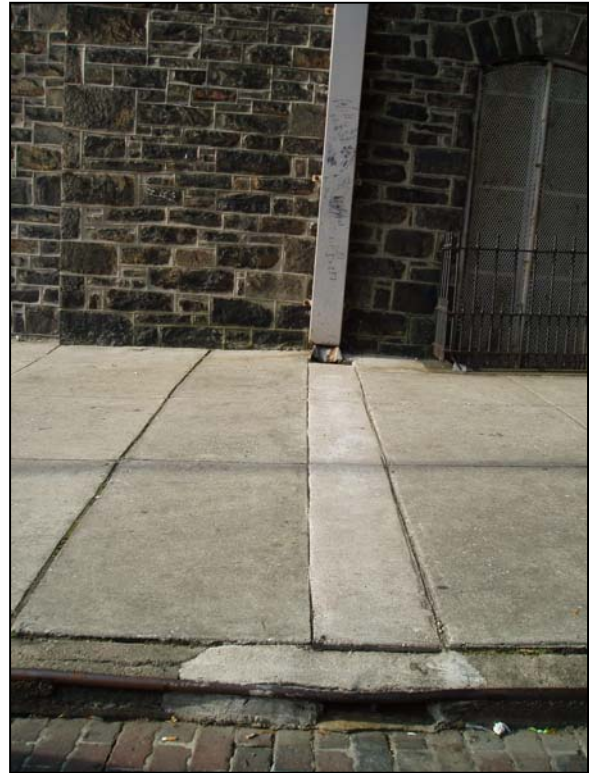
Figure 1: Downspout from St. Martin Church on Fayette.
