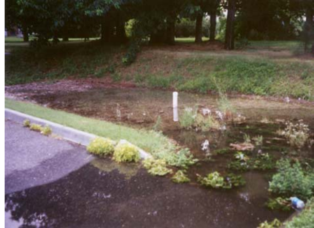
Figure 1: Failed Infiltration Trench
