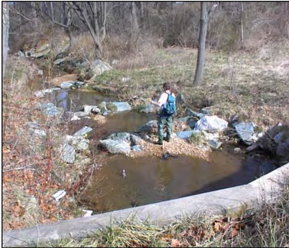
Figure 2: Use of a series of grade control structures downstream of a culvert
