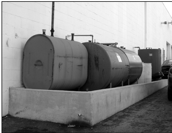
Figure 2: Secondary Containment of Storage Drums Behind a Car Repair Shop
