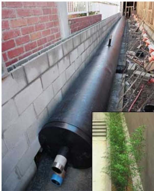
Rainwater cistern at NRDC's Santa Monica Office (inset photo after planter planting). Photo: NRDC.
