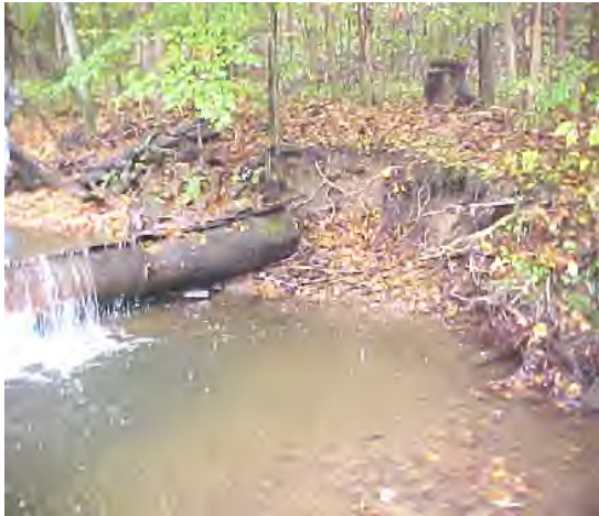
The arm of the K-Dam has collapsed resulting in bank erosion adjacent to the structure as well as further downstream.
