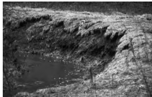
This steeply sloping bank has obvious and severe erosion.
