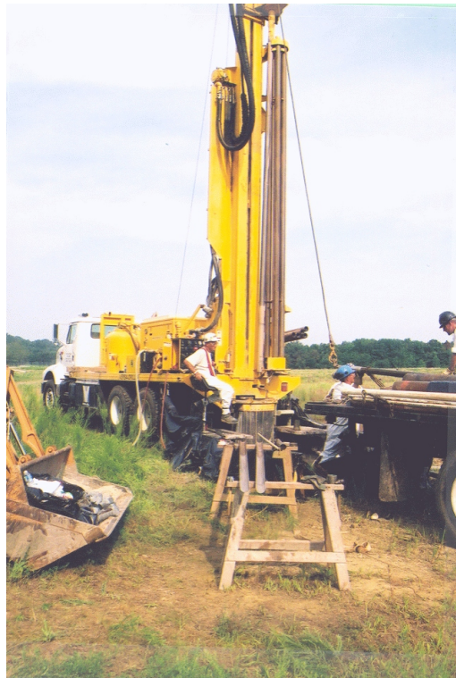
An air rotary drilling rig installing a new groundwater monitoring well at the Letart Landfill.
