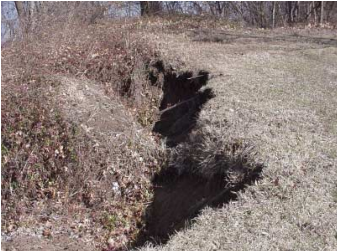
BANK COLLAPSING INTO THE KANAWHA RIVER
