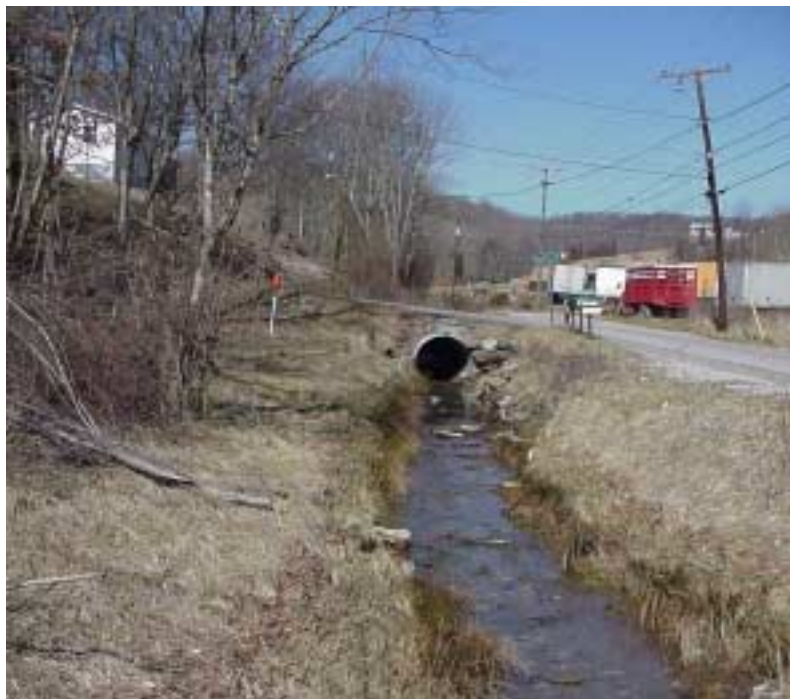
Typical culvert and road showing poor riparian buffer zone
