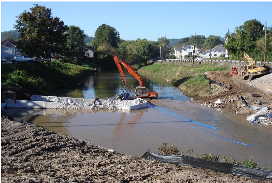
Figure 2-33. Example of Channel Alteration actively occurring due to an installation of sewage pipes across a stream channel.
