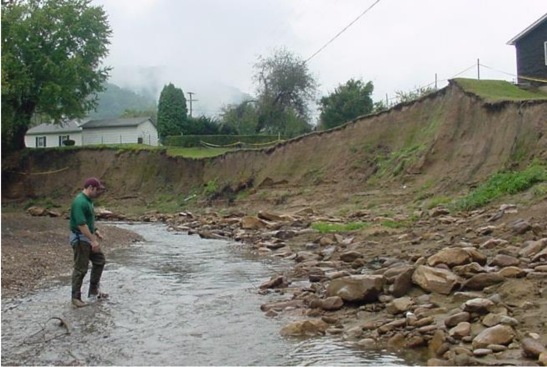
Figure 2-40. Example of heavy erosion (photo right).
