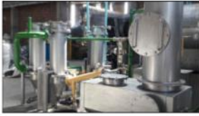
Figure 13. Photo A of a typical gas cleanup system in operation
