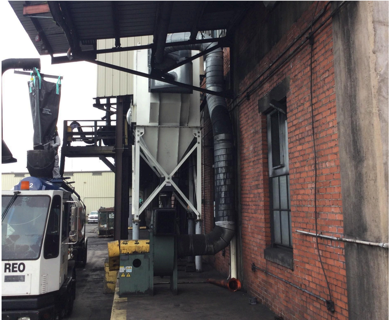
Figure 1 - 2S Tanker Truck Loading Baghouse and Emission Point 2E
