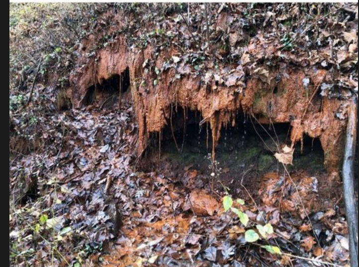
Collapsed and Draining Entry-Top of Main Slide
