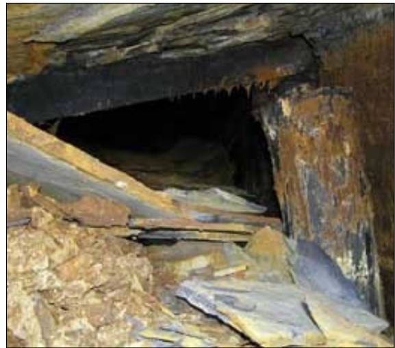
Collapsed mine portal
