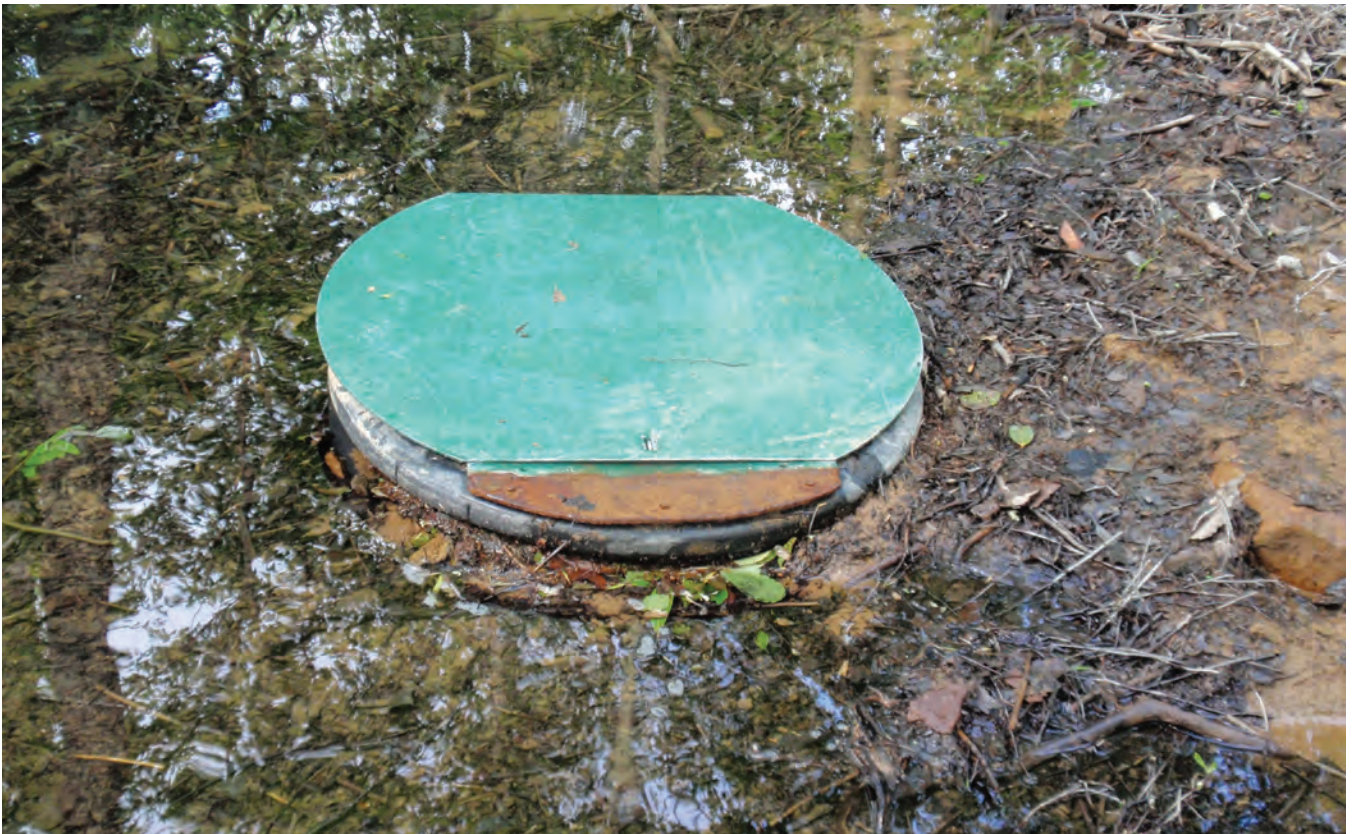
Debris clogging intake of the North Fork doser
