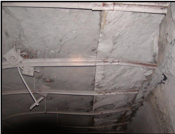
Underground Roof Crack
