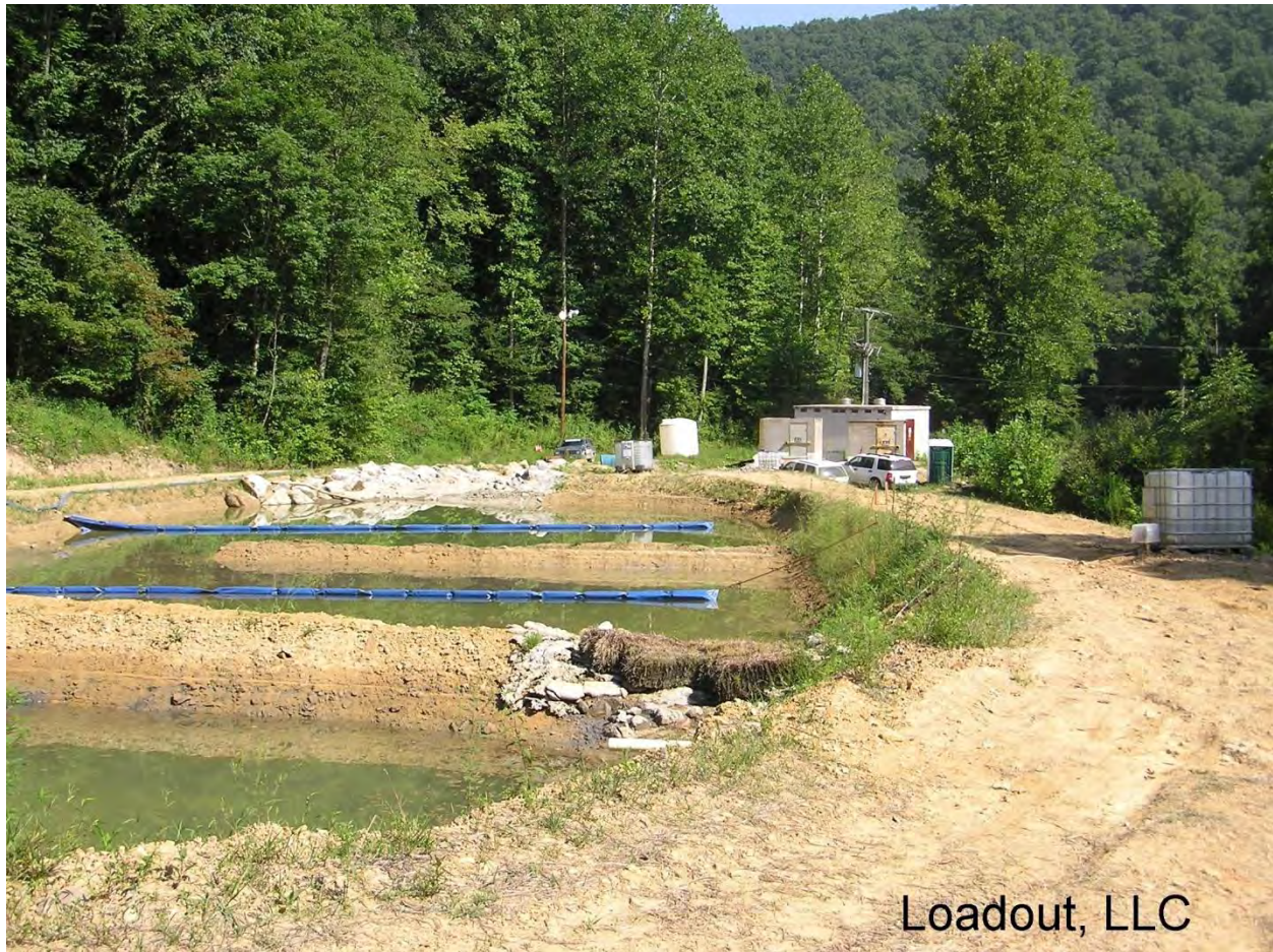
Picture LHAR-2: Picture shows the pump at LL-7 and the associated ponds.
