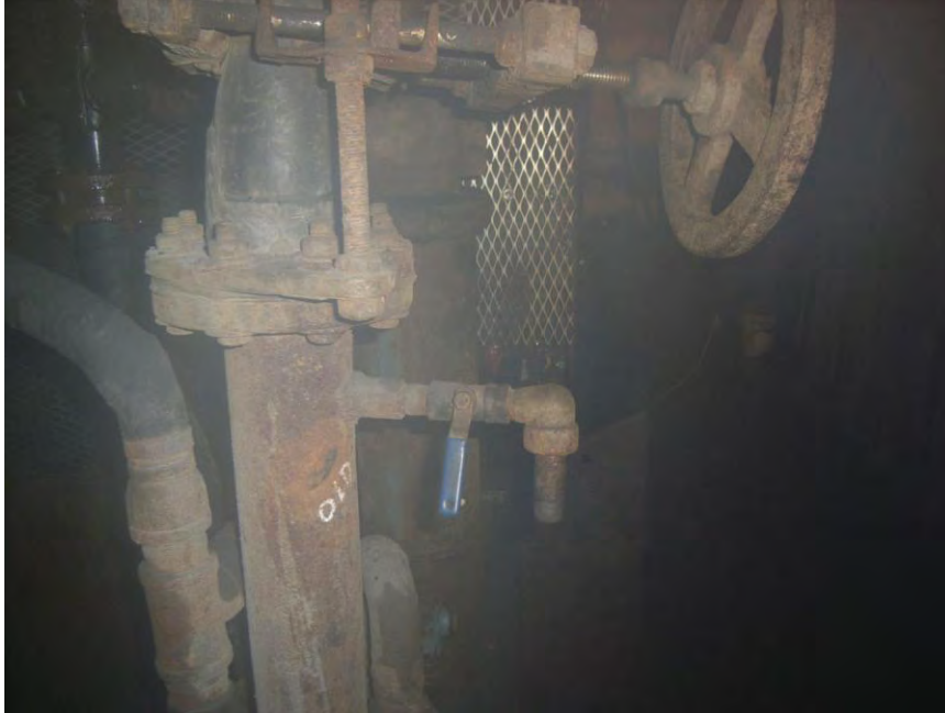
Picture LHAR-3: Loadout thickener decant pipe where slurry sample is taken.
