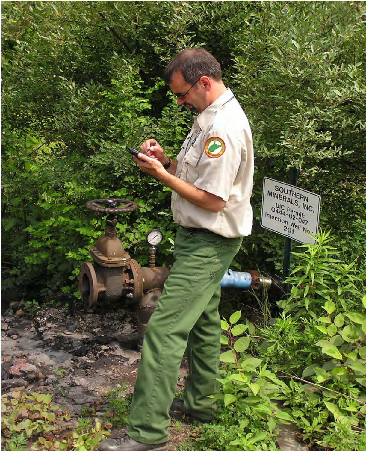
Figure 28 UIC-201 active slurry injection site.
