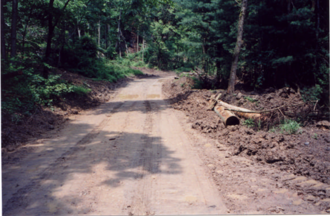
Picture 12 – Uninstalled stream crossing pipes on an active timber haulroad.
