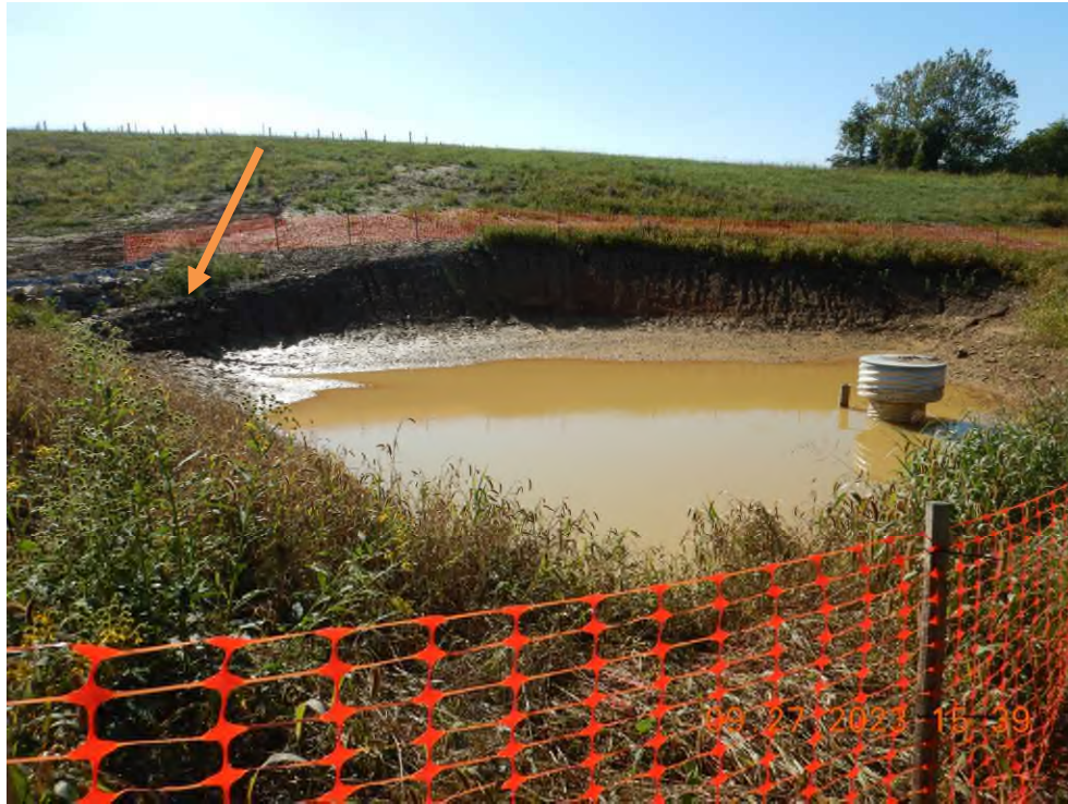
Sediment Pond 6 has unstable inlet.
