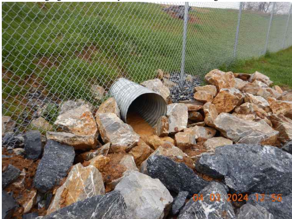
Outlet 6 discharging sediment laden water.
