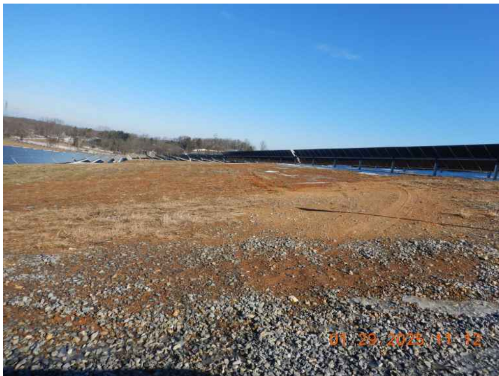
An unstabilized area of the project.
