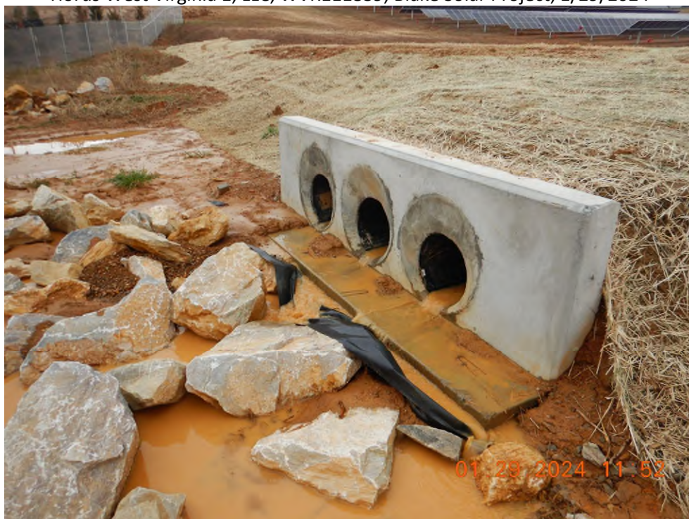
Basin 11 discharging offsite.
