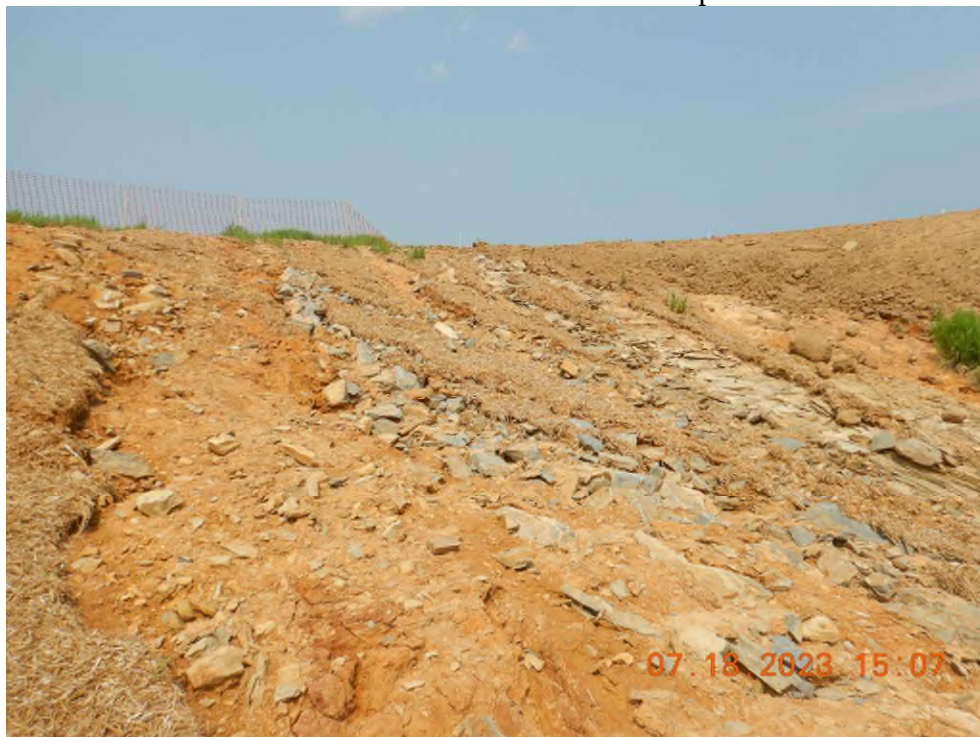
Erosion rills need stabilization.
