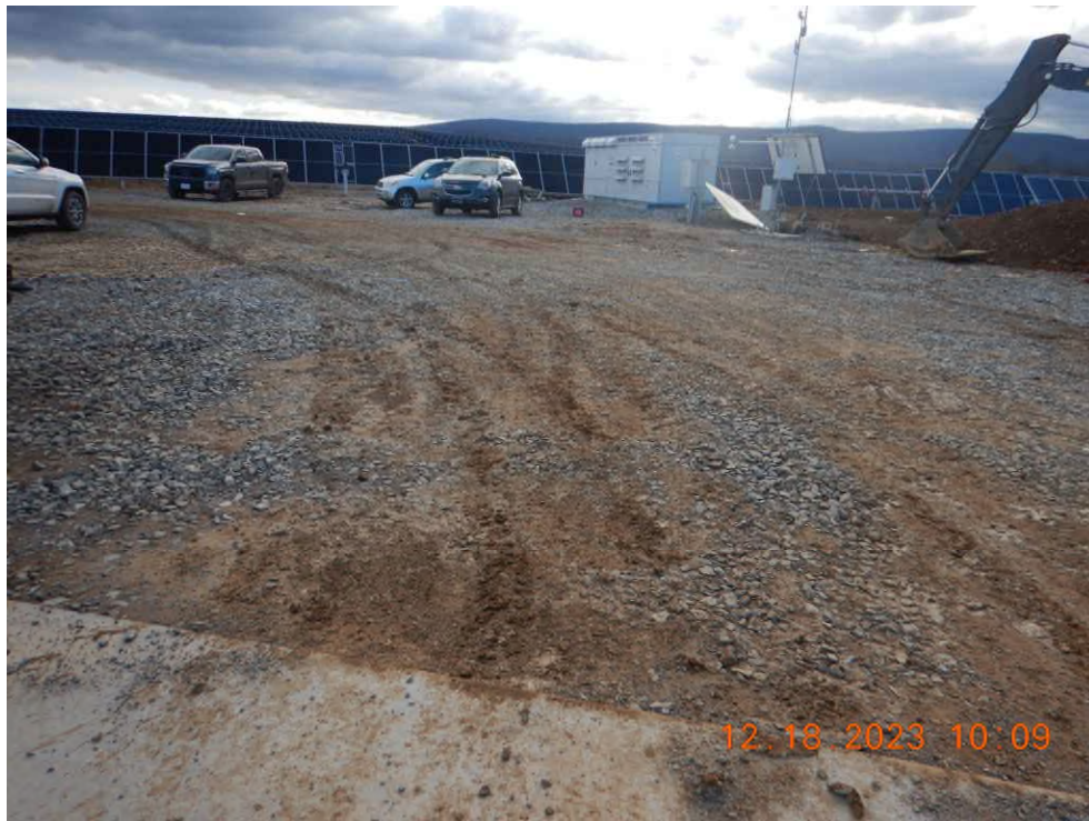
Construction entrance needs stabilized
