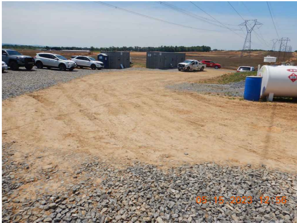
Unstabilized construction entrance.
