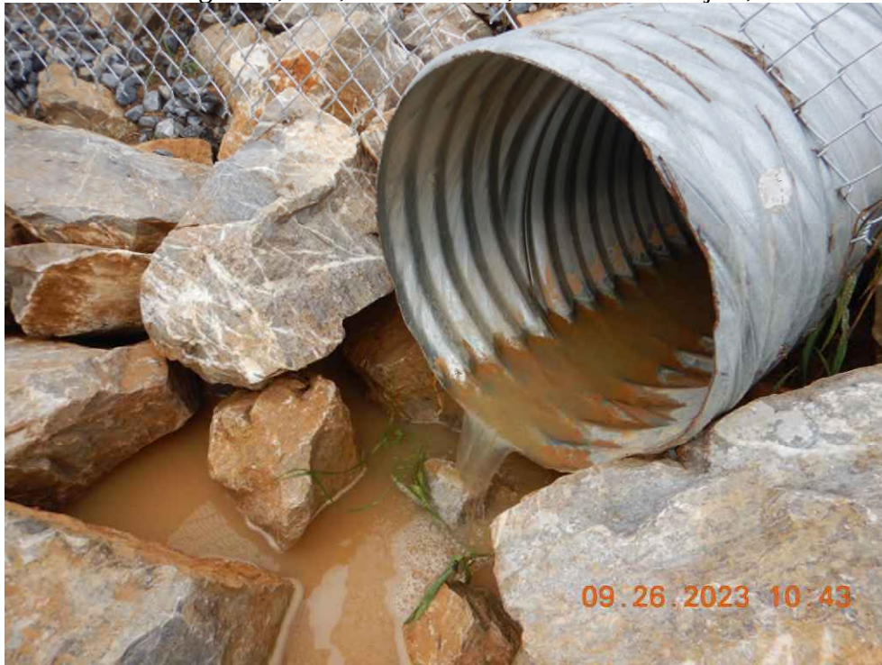
Sediment laden water discharging from Sediment Basin 6.
