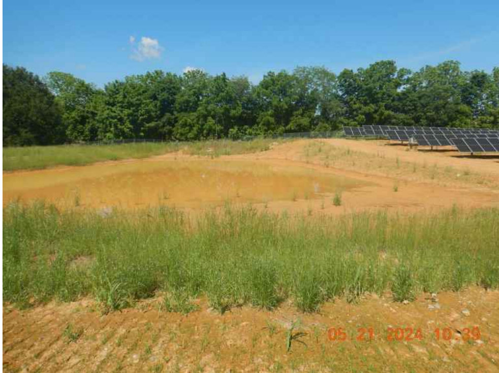
Unstabilized area above Sediment Basin 8.
