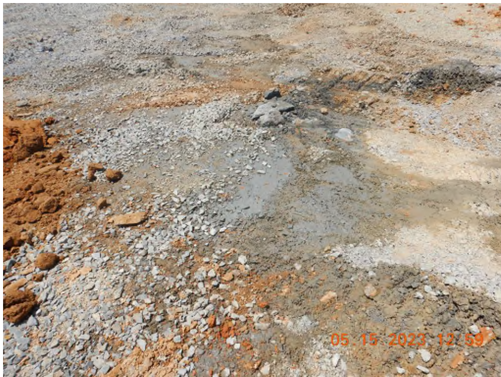
Concrete washout is not being used properly.
