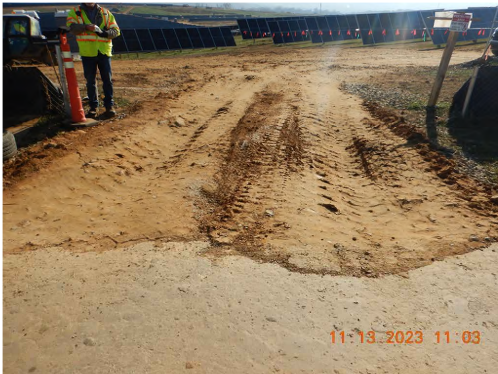
Unstabilized construction entrance.
