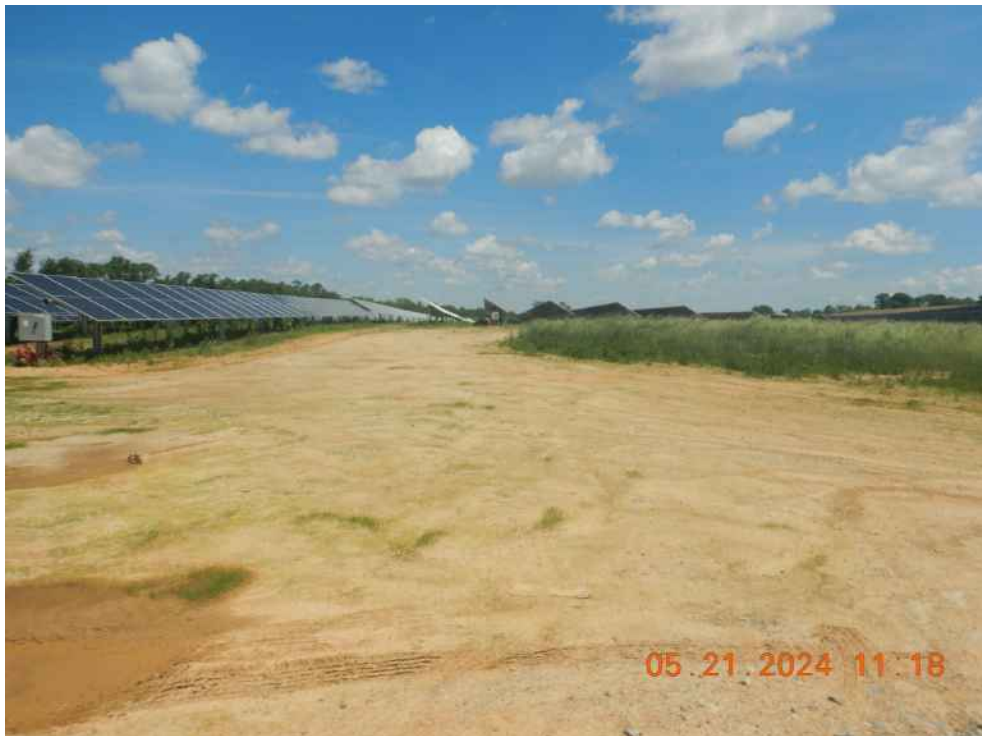
Unstabilized area above Sediment Basin 10.
