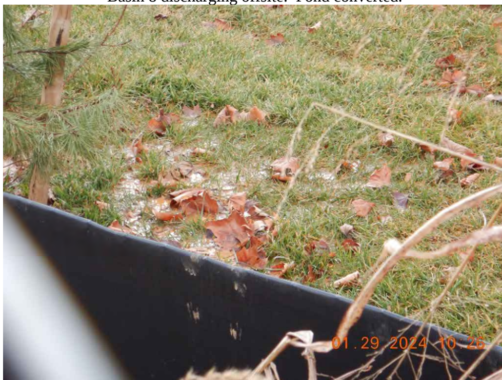
Basin 8 discharging offsite.
