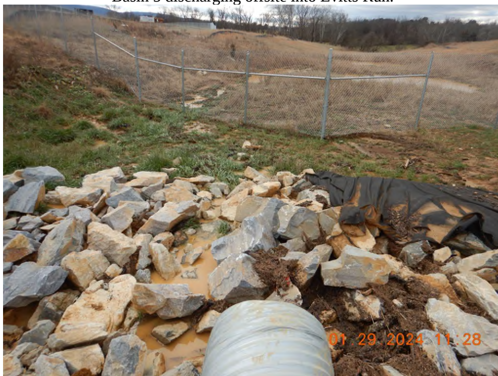
Basin 13 discharging into Evitts Run.
