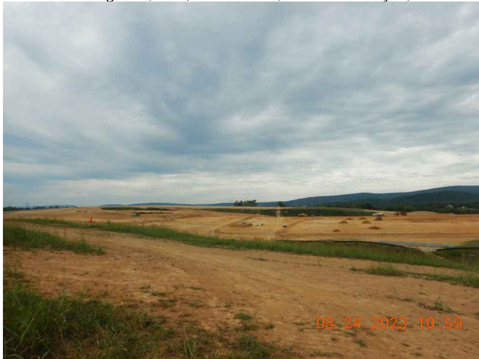
Area that lacks stabilization.
