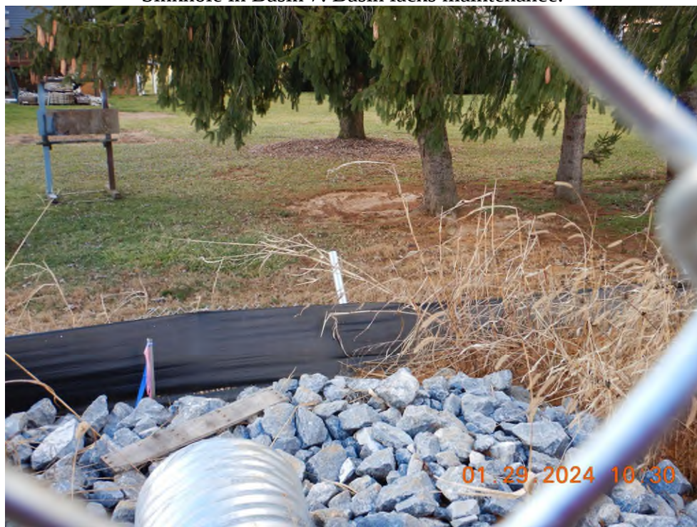
Basin 7 discharging offsite.
