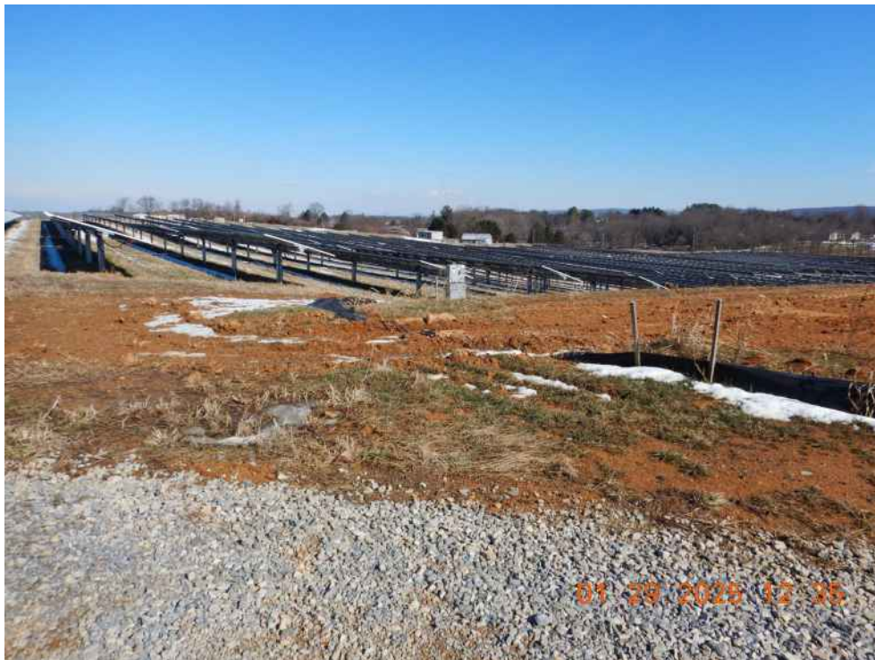
An unstabilized area of the project.
