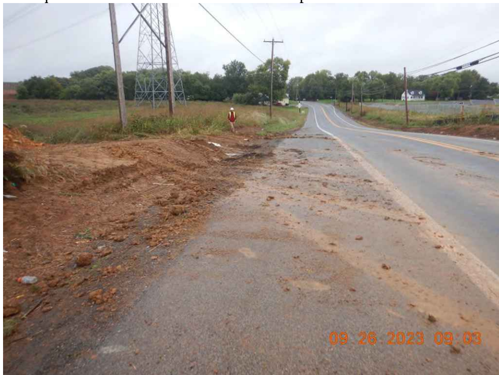
Unstabilized construction entrance.
