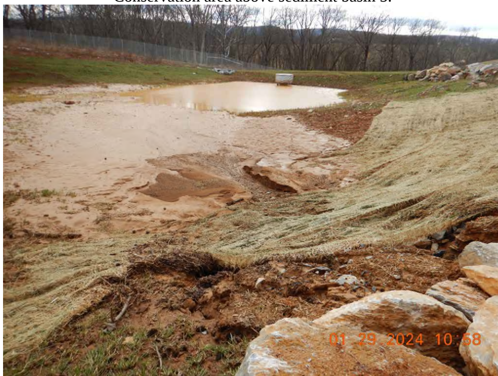
Basin 5 is in need of maintenance.
