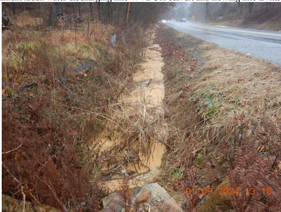
Sediment laden water following WVDOH ditchline into Evitts Run
