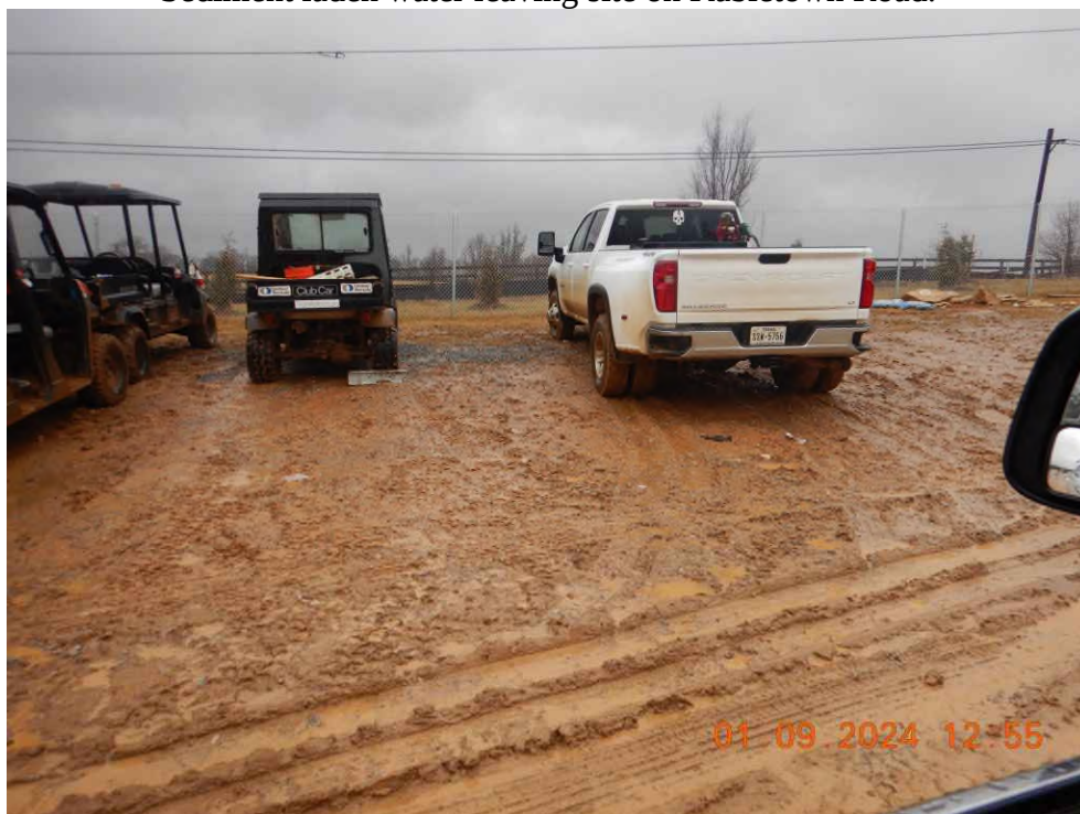
Unstabilized construction entrance by Entrance 2 Kabletown Road
