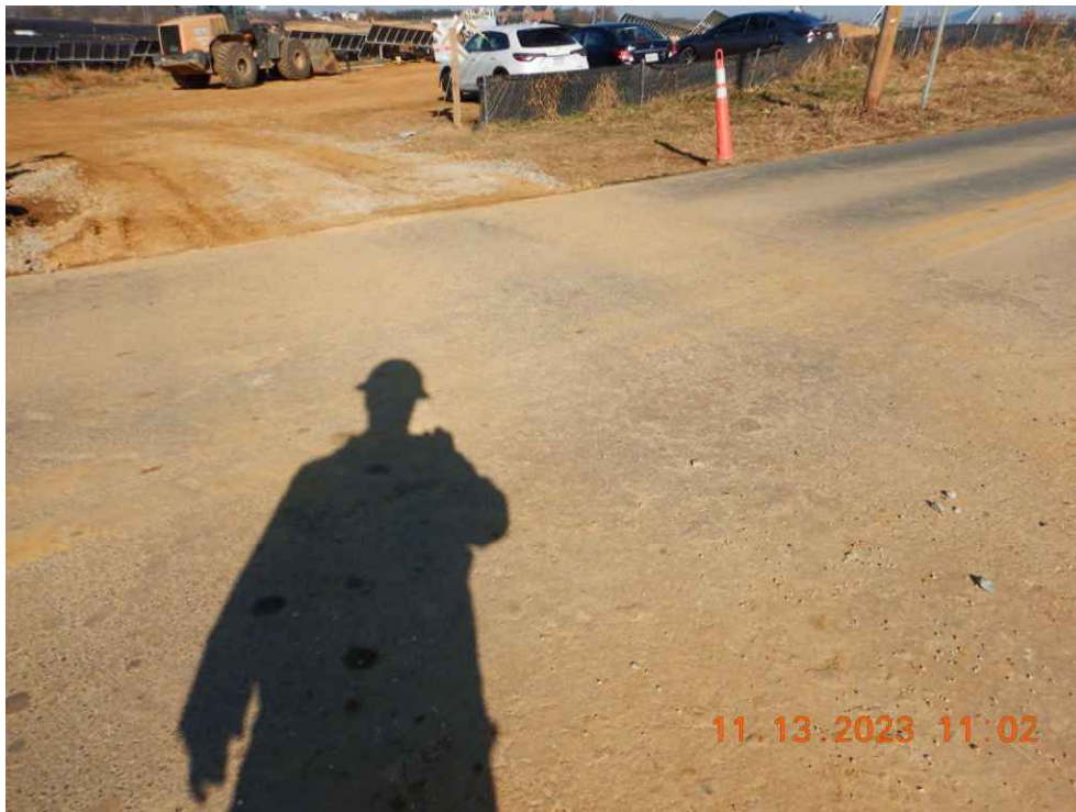
Unstabilized construction entrance.
