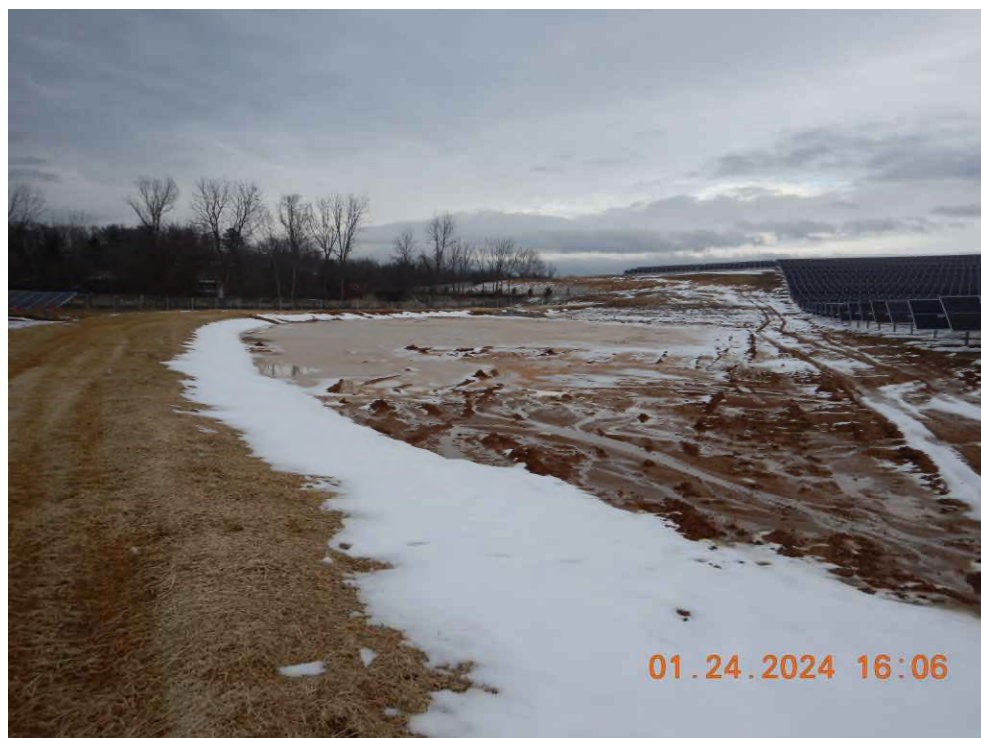
Pond 2B that has been installed and is discharging sediment laden water offsite.
