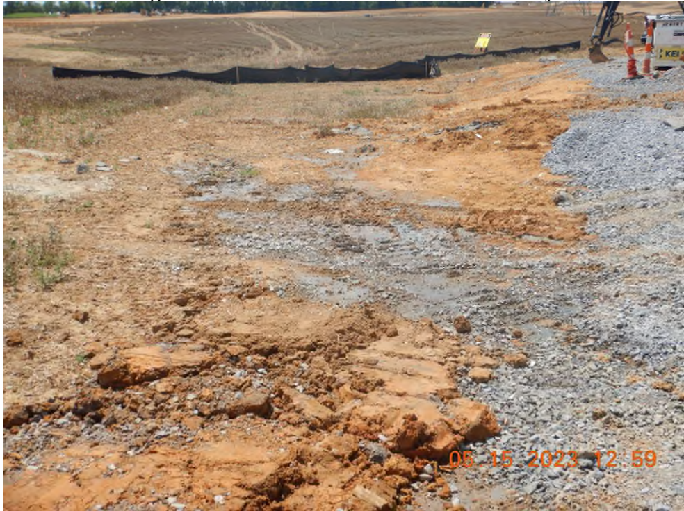
Concrete washout not being used.
