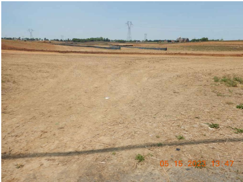
Construction entrance needs stabilization.
