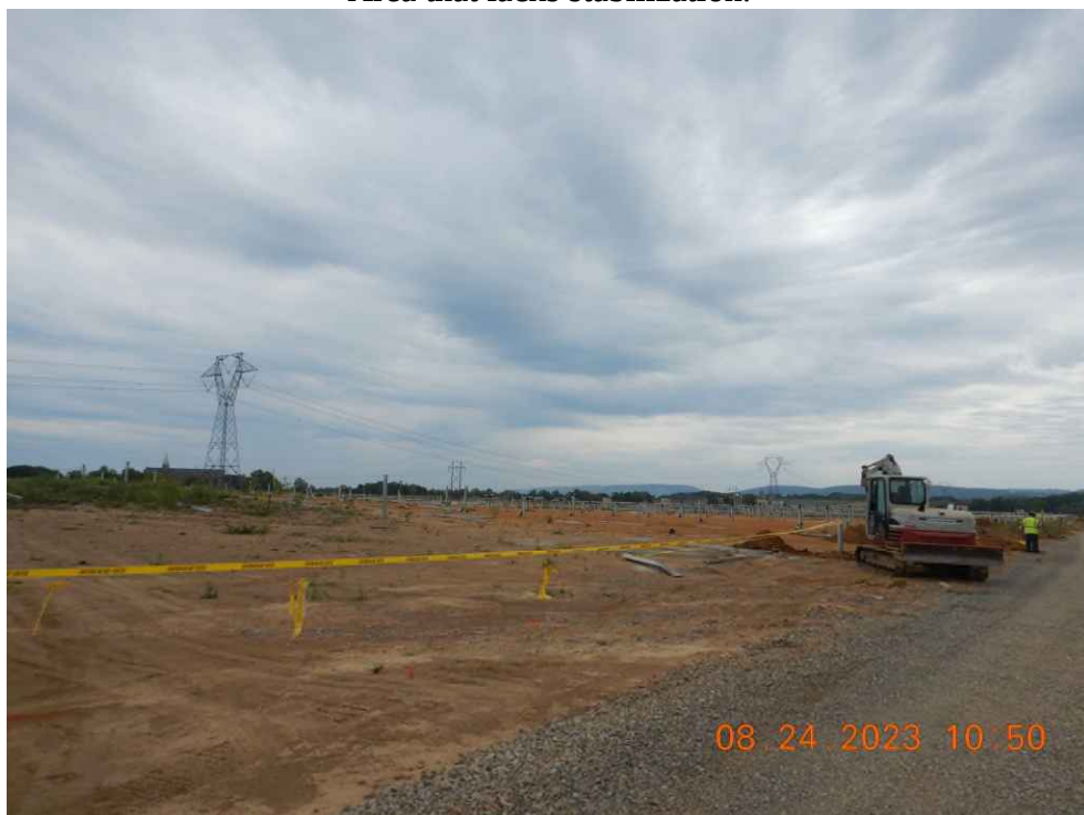
Area that lacks stabilization.
