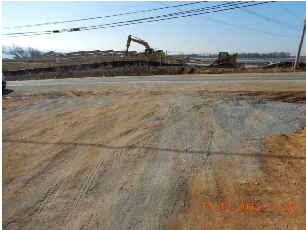
Unstabilized Construction Entrance.
