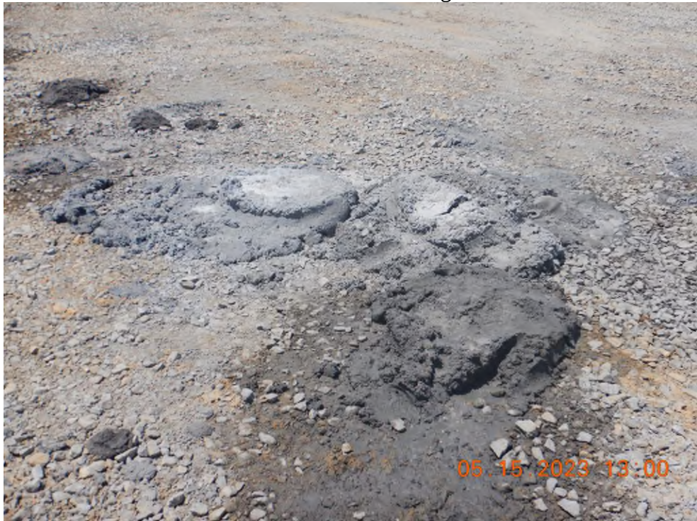
Concrete washout not being used.
