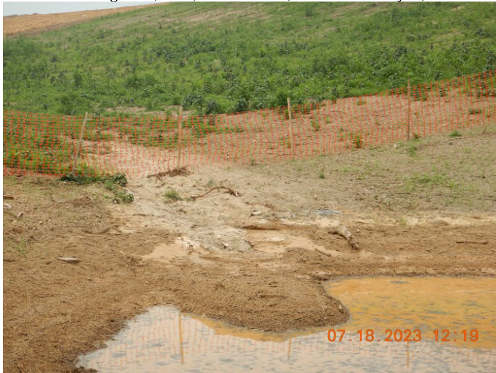
Unstable inlet to Sediment Basin 6.
