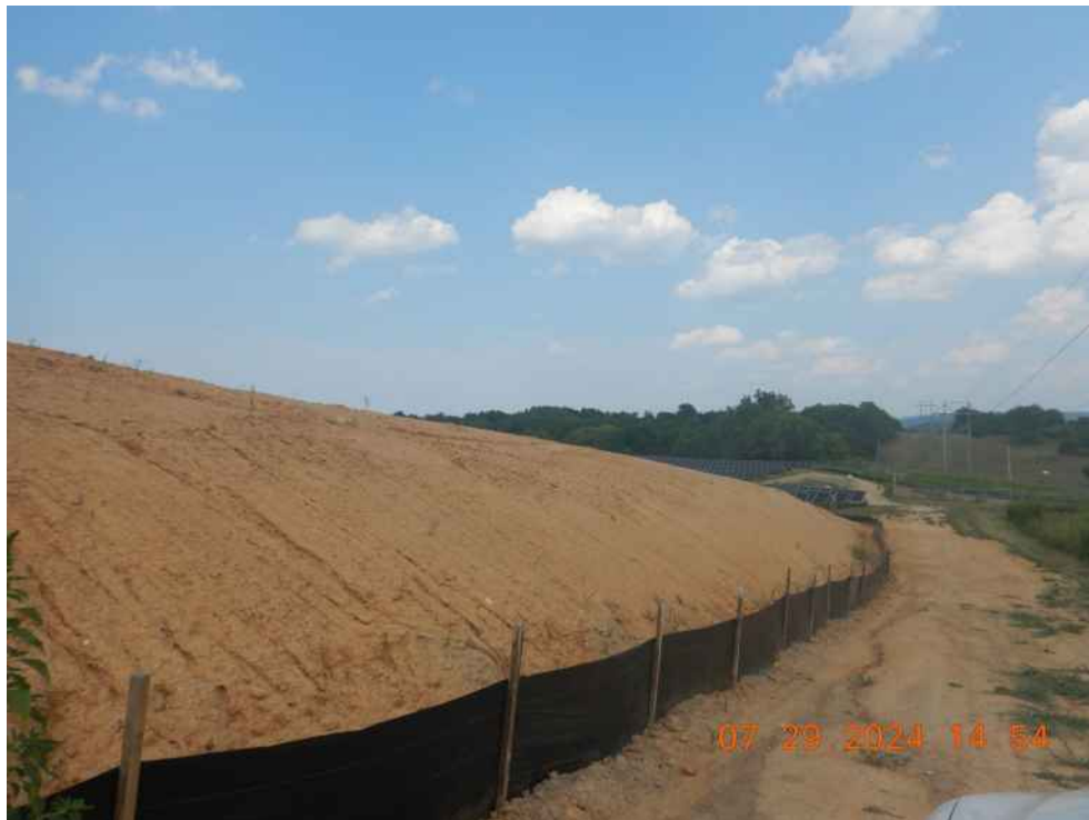
An unstabilized soil stockpile. Sediment trap 2 area.
