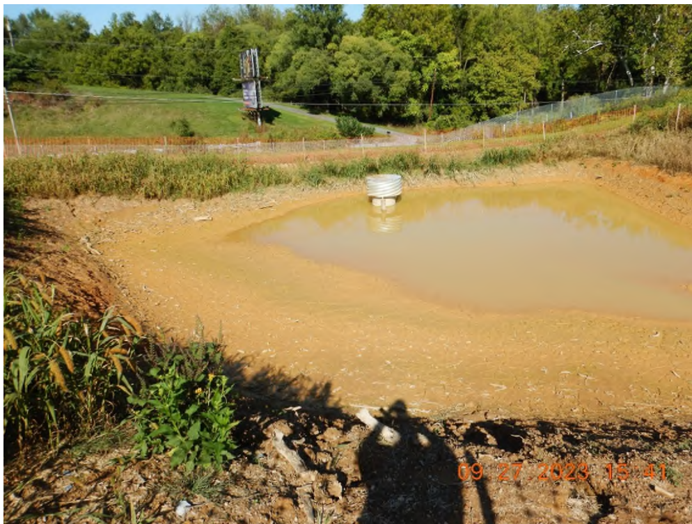
Sediment Basin 6 with accumulated deposits.
