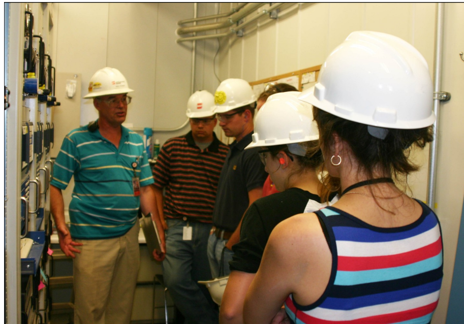
Reid Strader, (far left), an engineer at the John Amos Power Plant near Winfield, talks to a group of Division of Air Quality interns during a visit to a shelter that houses gas analyzers.
