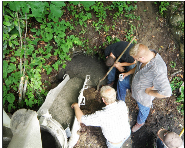
Workers seal up one of two portals that were used by Raleigh County teen-agers to explore an abandoned coal mine.
