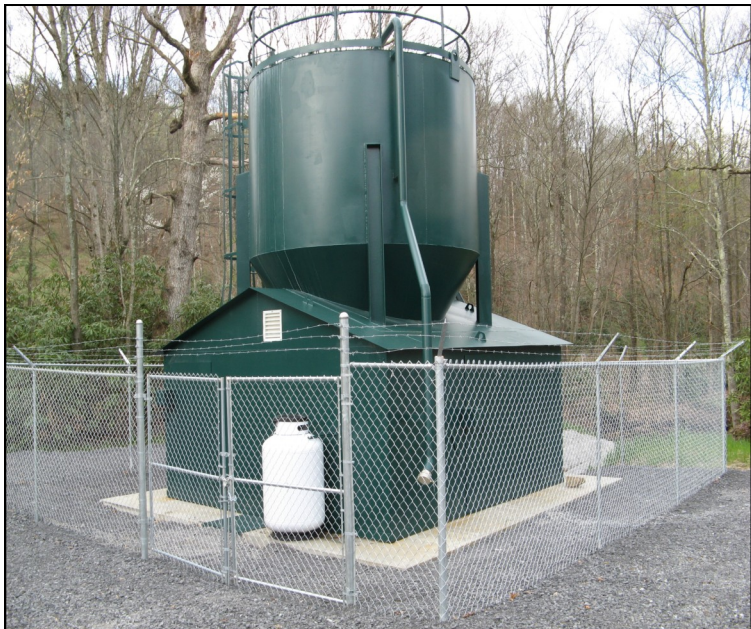
Below, Abandoned Mine Lands Chief Eric Coberly, left, and local watershed president Leroy Stanley officially activate one of four dosers that will treat acid mine drainage on Three Fork Creek in Preston and Taylor counties. The Pell School Road Site doser is pictured above. The AML project cost $750,000.
