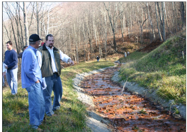
Brady Gutta (right), project manager with the West Virginia University National Mine Land Reclamation Center, speaks with state, county and local officials during a tour of Lambert Run’s restoration projects. Above, Gutta describes how an open limestone channel treats mine drainage.
