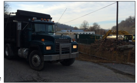
Truckloads of soil from the former Freedom Industries site are being taken to the Charleston Landfill for proper disposal.
