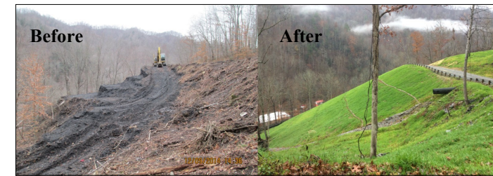
AML&R's projects included this one at the Black Eagle #2 refuse pile in Wyoming County. It's one of dozens of projects that eliminated health and safety hazards for citizens living in mining areas of West Virginia.
