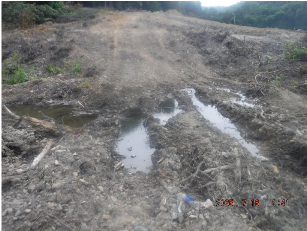
Photo # DSCF5366: Sediment deposits from equipment crossing in UNT Mahan Run at or near N 40° 20.5848', W 80° 35.7501'.
