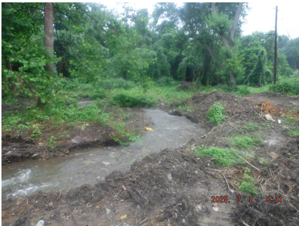
Photo # DSCF5060: No E&S controls installed
