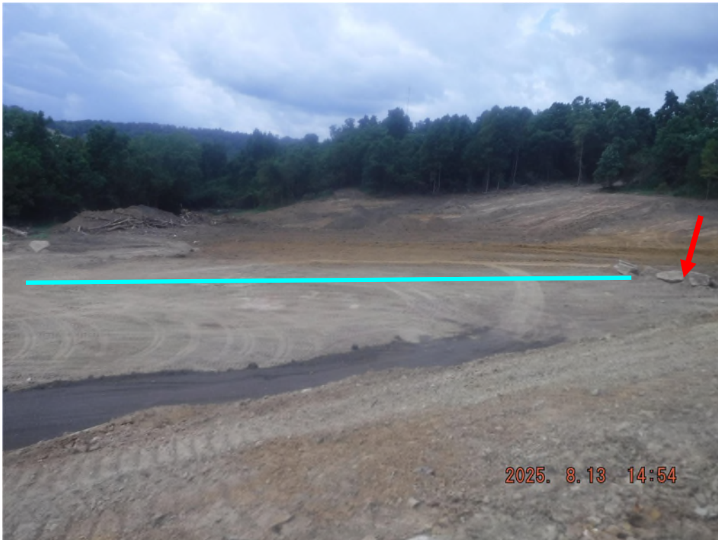
Photo # DSCF6177: Red arrow showing location of culvert inlet for UNT Mahan Run at or near N40° 20.6166', W80° 35.7455'. Blue line is approximate 400' path of culvert under fill material
