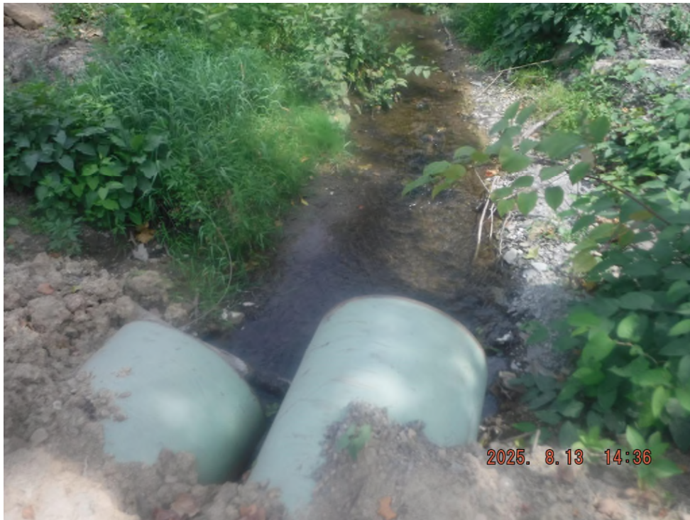
Photo # DSCF6156: Fill and culvert crossing at or near N 40° 20.5392', W 80° 35.6935' creating conditions not allowable in Mahan Run.
