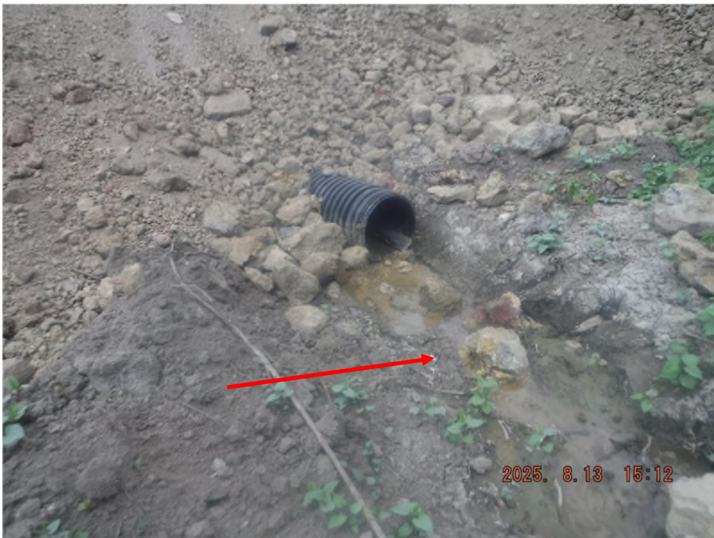
Photo # DSCF6238: Culvert outlet of UNT Mahan Run at or near N40° 20.5509', W80° 35.7524' with sediment deposits downstream of the culvert
