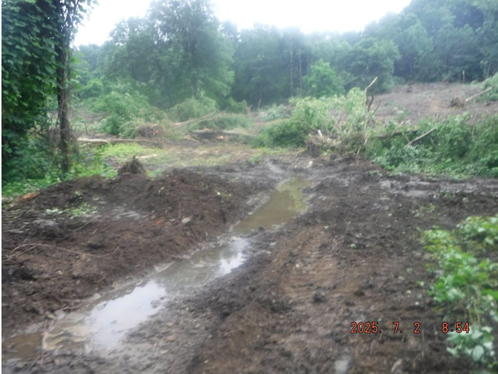
Photo # DSCF5092: Sediment deposits in UNT Mahan Run at or near 40.343044, -80.595879
