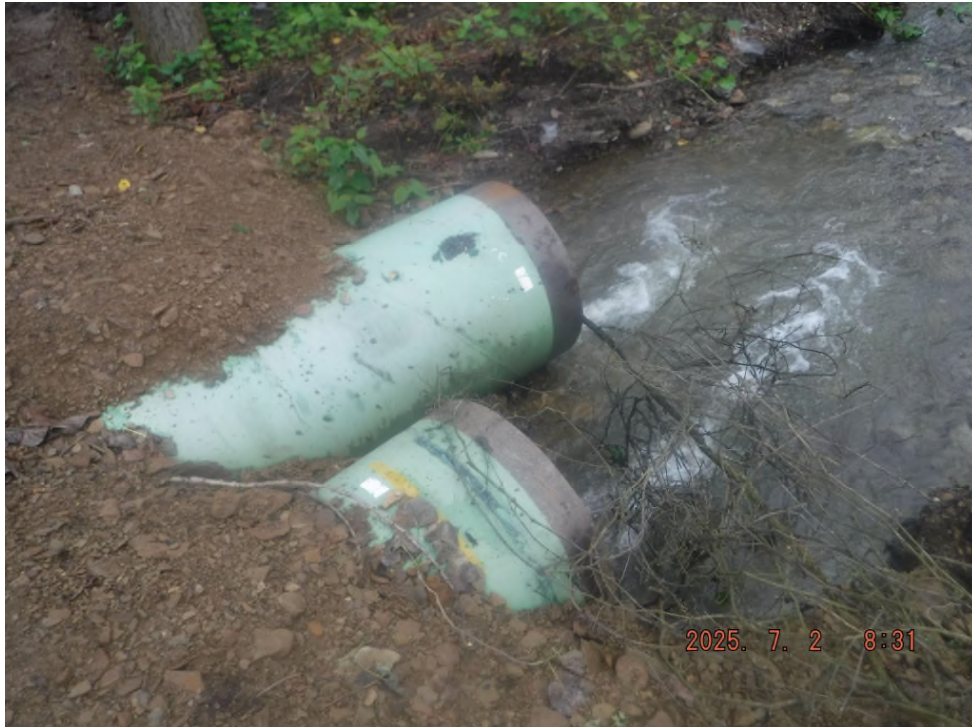
Photo # DSCF5058: Sediment placed in Mahan run at or near N 40° 20.5392', W 80° 35.6935' for a stream crossing (downstream view)
