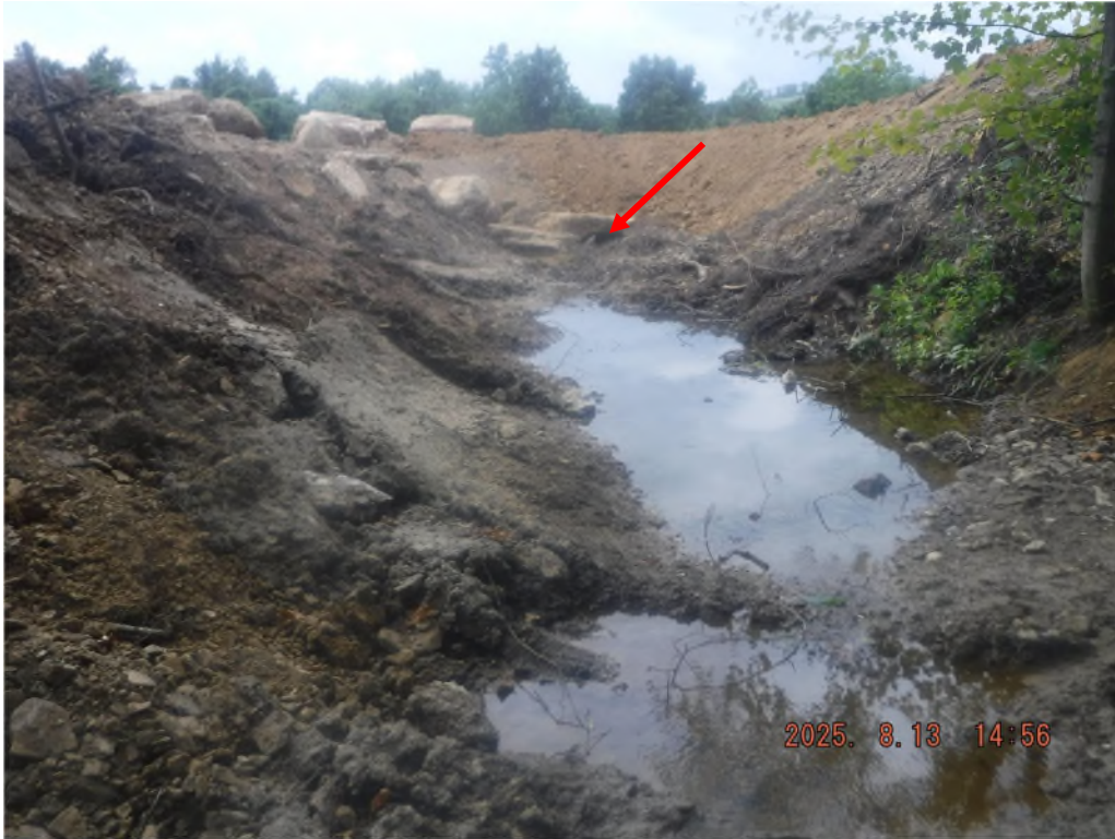
Photo # DSCF6185: Sediment deposits in UNT Mahan Run at or near N40° 20.6255', W80° 35.7453'. Red arrow shows culvert inlet and fill material at or near N40° 20.6166', W80° 35.7455'.
