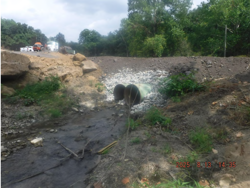
Photo # DSCF6154: Fill and culvert crossing at or near N 40° 20.5392', W 80° 35.6935' creating conditions not allowable in Mahan Run.
