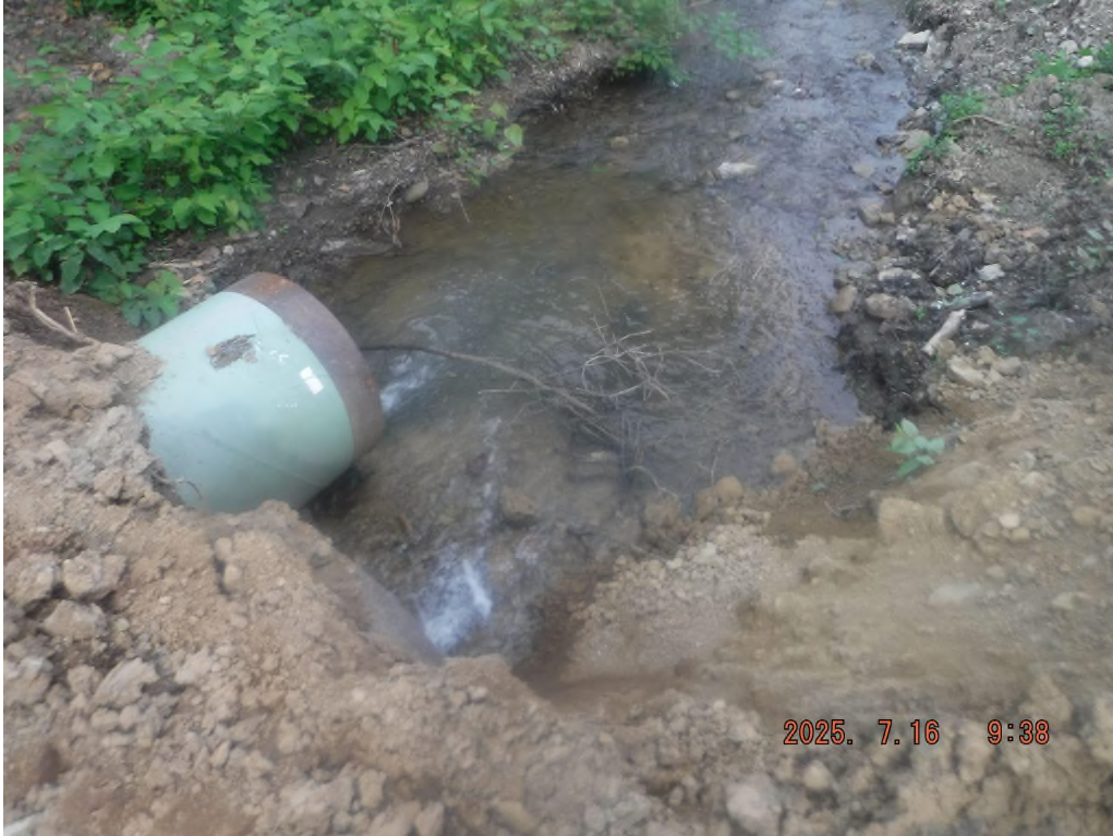
Photo # DSCF5357: Fill, culvert crossing, and sediment deposits in Mahan Run at or near N 40° 20.5392', W 80° 35.6935'.
